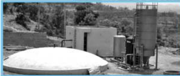
INDION® Water Treatment Plant
