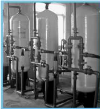
INDION® Solar Based Community Plant for Arsenic Removal
