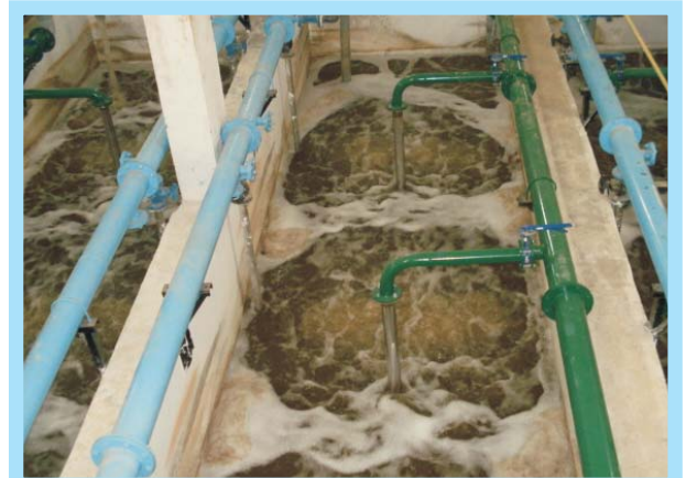
Sewage Treatment & Recycle
